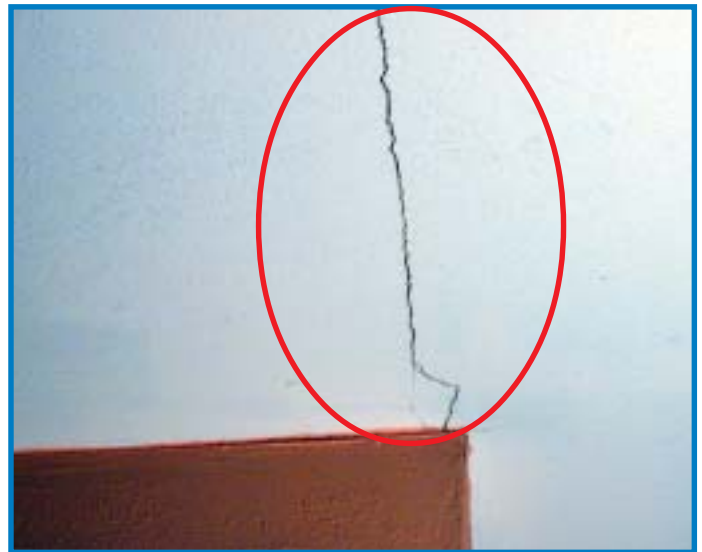
Drywall cracking at the ceiling
