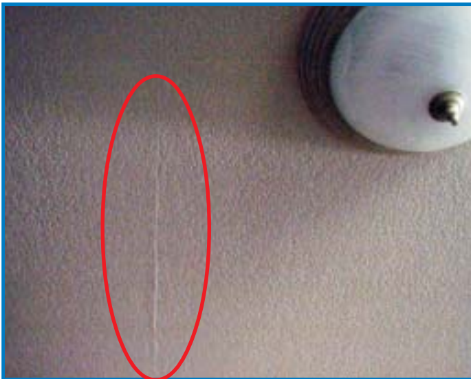
Drywall crowning at the ceiling
