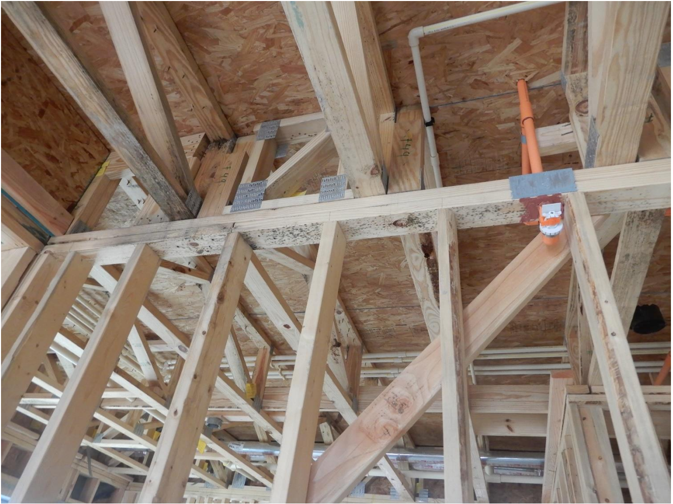
Photo 2: Mold on Installed Wood Members
